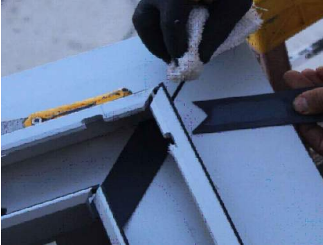
Clean units surfaces
